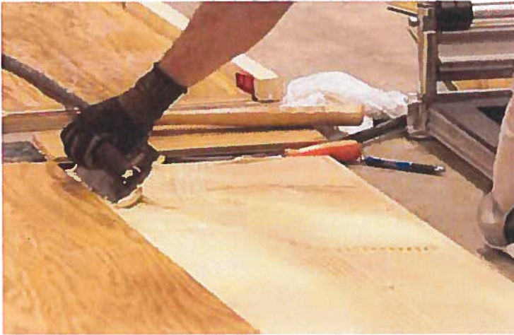
Bent wrist to trowel adhesive: Use inline trowel or angled handle traditional trowel (avoids flex/extension but increases ulnar deviation).
