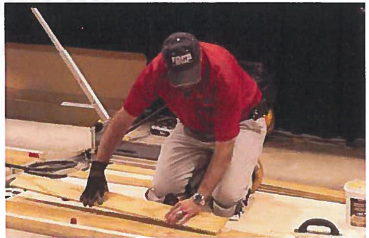
Much of the pain and suffering associated with hours of bending or kneeling, lifting heavy material and tools, can be alleviated and/or diminished with ergonomics.
